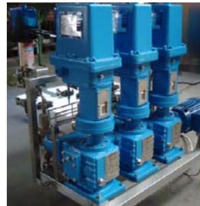
The dosing unit is installed on a stainless frame.
